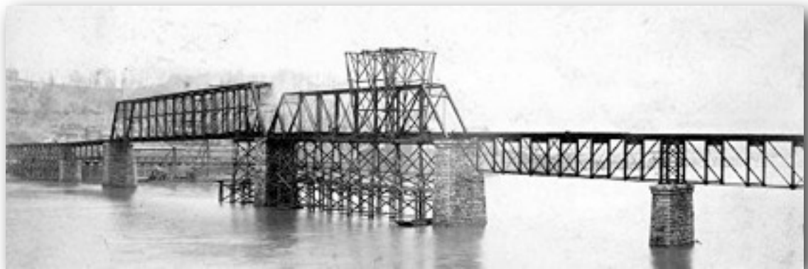
The Monongahela Connecting Railroad Bridge being constructed in 1877 (subsequently redesigned and known today as the Hot Metal Bridge).
